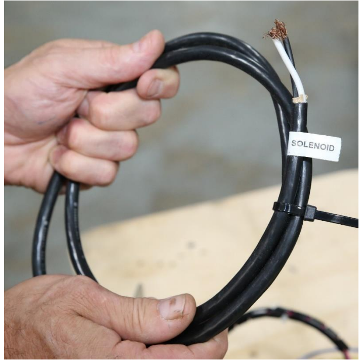
The Solenoid Cable is wrapped up and labeled. This is for a 208/240VAC Solenoid Valve Coil.
